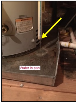
Leaking pressure valve
