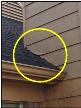
Damaged siding/ fireplace
