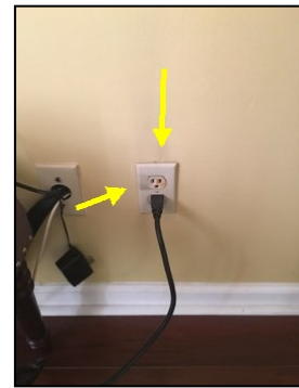
Heat/ arc markings
