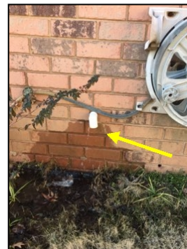
Water coming from water heater
