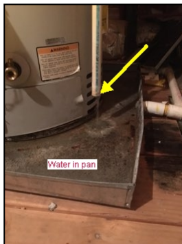
Leaking pressure valve
