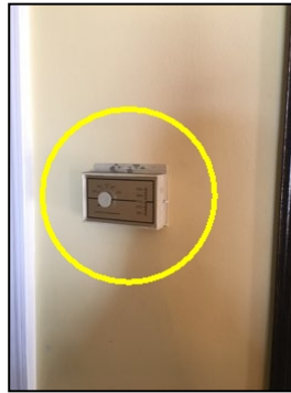
T-stat/ missing front and reading 50deg
