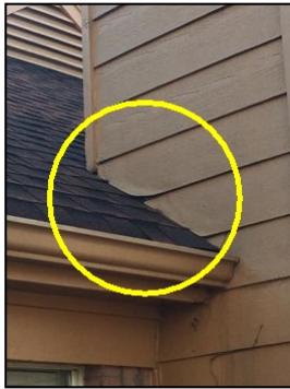
Damaged siding/ fireplace
