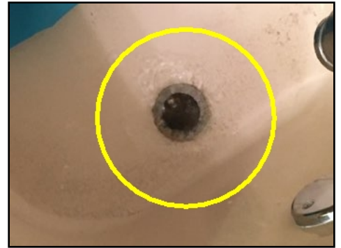
Missing stopper/ hall bath
