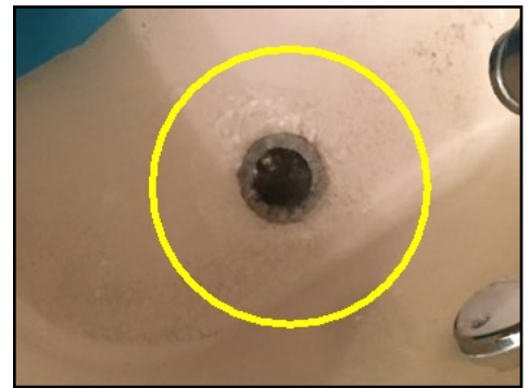
Missing stopper/ hall bath
