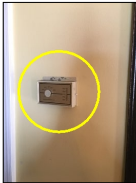
T-stat/ missing front and reading 50deg
