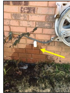
Water coming from water heater
